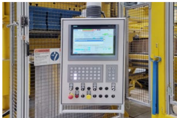
Control panel for the press plant and the brick placing robot
